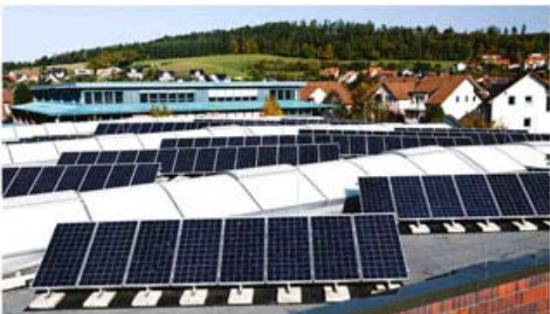
SWR - GH - Photovoltaik 009.jpg
