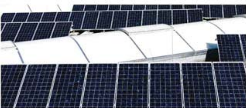
SWR - GH - Photovoltaik 015.jpg
