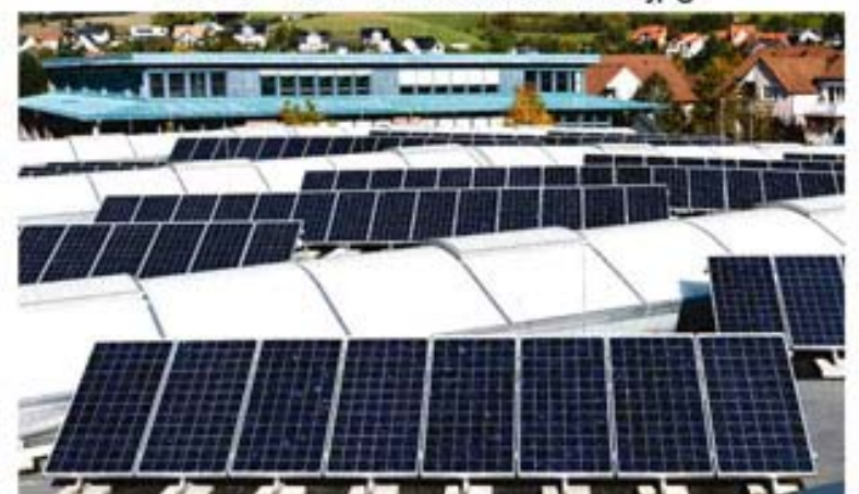
SWR - GH - Photovoltaik 011.jpg
