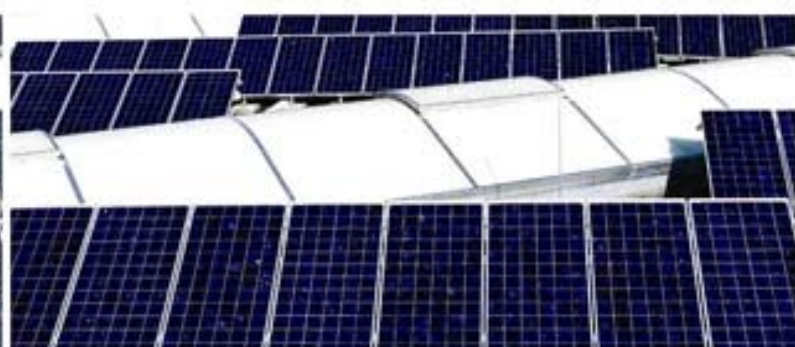
SWR - GH - Photovoltaik 016.jpg
