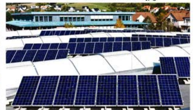
SWR - GH - Photovoltaik 012.jpg
