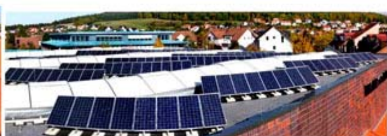
SWR - GH - Photovoltaik 004.jpg
