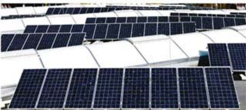
SWR - GH - Photovoltaik 013.jpg
