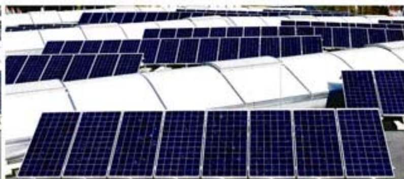
SWR - GH - Photovoltaik 014.jpg
