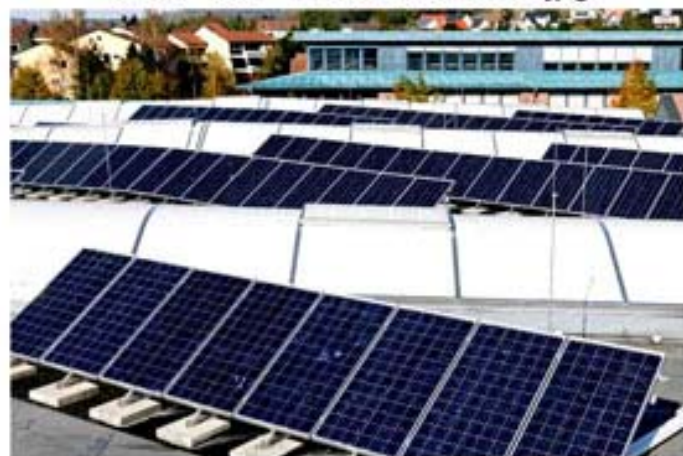
SWR - GH - Photovoltaik 008.jpg
