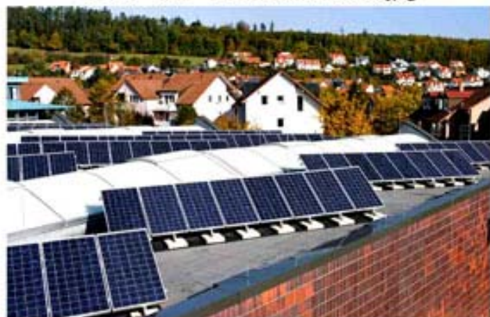
SWR - GH - Photovoltaik 007.jpg
