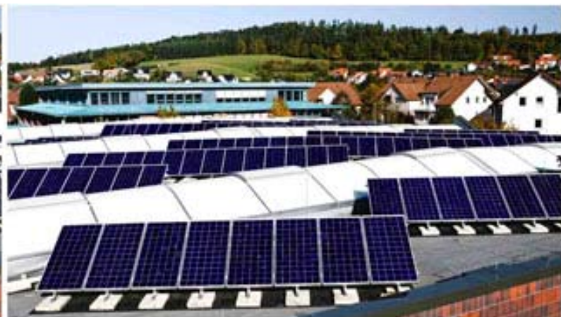
SWR - GH - Photovoltaik 010.jpg
