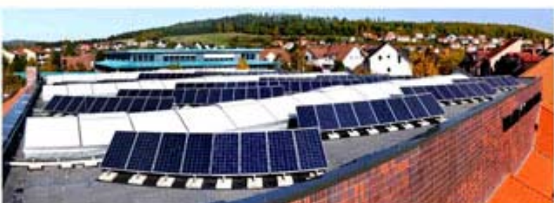
SWR - GH - Photovoltaik 003.jpg
